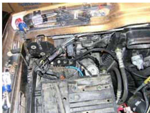
Battery tray back in with no more problems.
